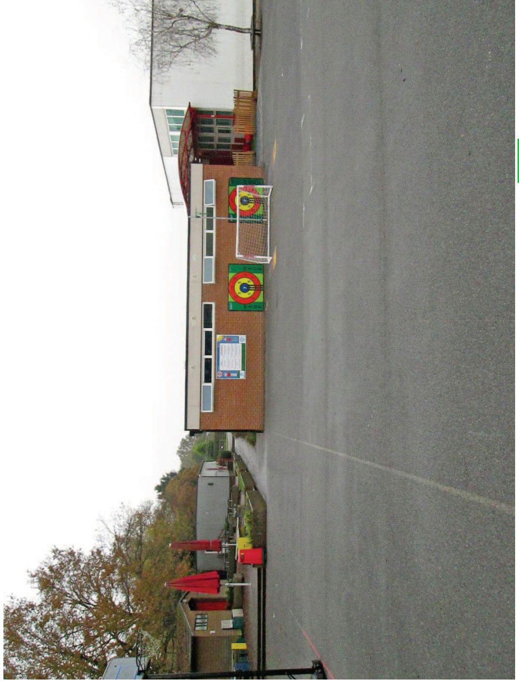
Figure 2 : View looking west from location of teaching block, showing part of hall on right and a modular building to be removed
