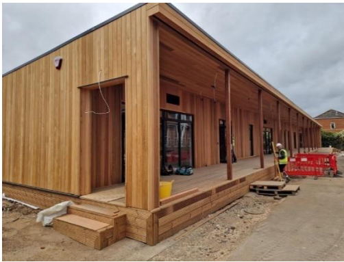
Image of the exterior of the new timber clad three classroom SEN Unit block at Stepgates Community School nearing completion in Chertsey.
